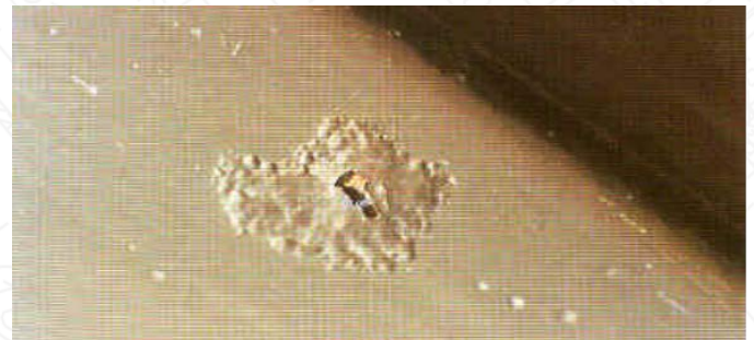
Image 2: Formation of bubbles due to under-rusting
