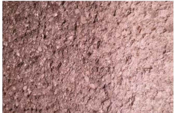
Friable and worn out surface
