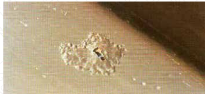
Image 2: Formation of bubbles due to under-rusting
